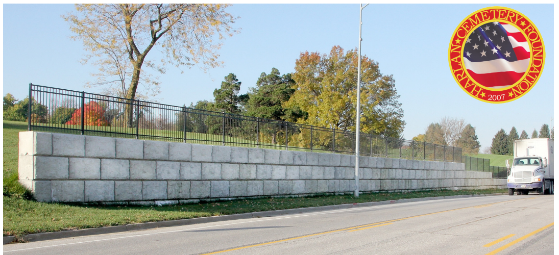
Just one of the new retaining walls with new fencing at the Harlan Cemetery.
